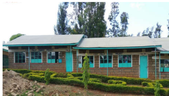
Two classrooms constructed in the same School at a total cost of KShs 500,000. The classrooms were complete and in use
